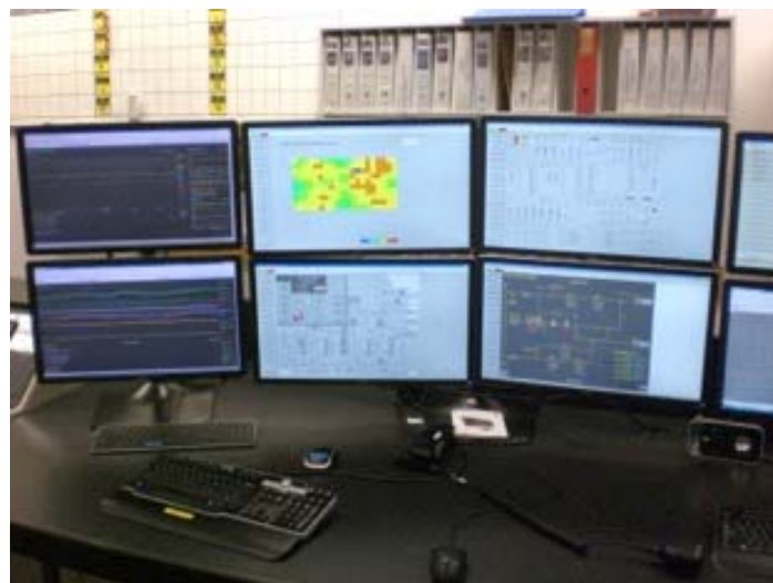
Figure 10: TGM DCS view installed in a control room.
