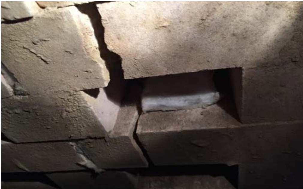
Figure 10 - Unsupported Brick Failure
