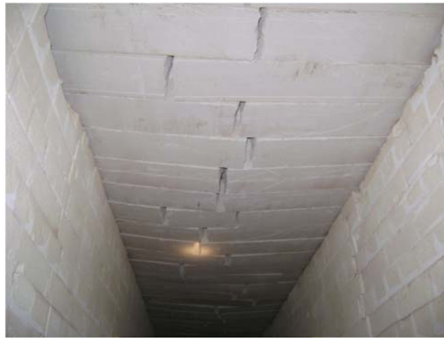
Figure 8 - Tunnel Lid Thermal Stress Failure Mode
